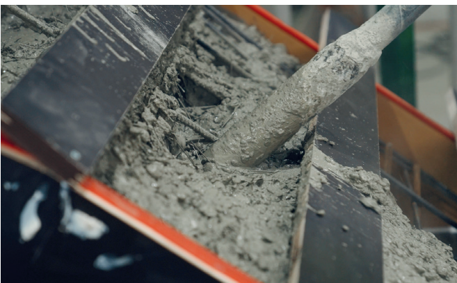
The installation of the fresh concrete with the Stabils fibre proves to be very simple. The fibres show a very homogeneous distribution in the fresh concrete and no tendency to clumping.
