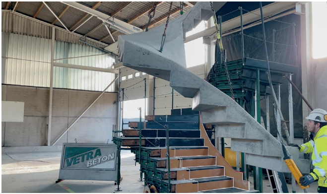
Lifting of the CO 2 -reduced precast concrete staircase. By using a combination reinforcement, the staircase can be manufactured very material-efficiently.
